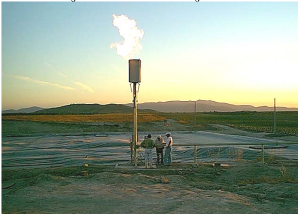
Figure 3: Methane combustion at Digester's Flare
